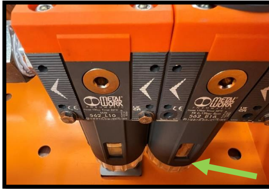
Fig.7: Drainage point below the regulator/filter unit.
